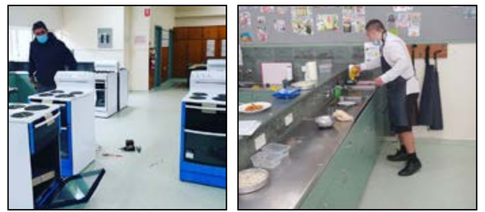
The VCAL class cooking with the newly installed replacement ovens
